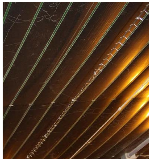
Figure 3. Corona lines for EPI system near roof of poultry house.
