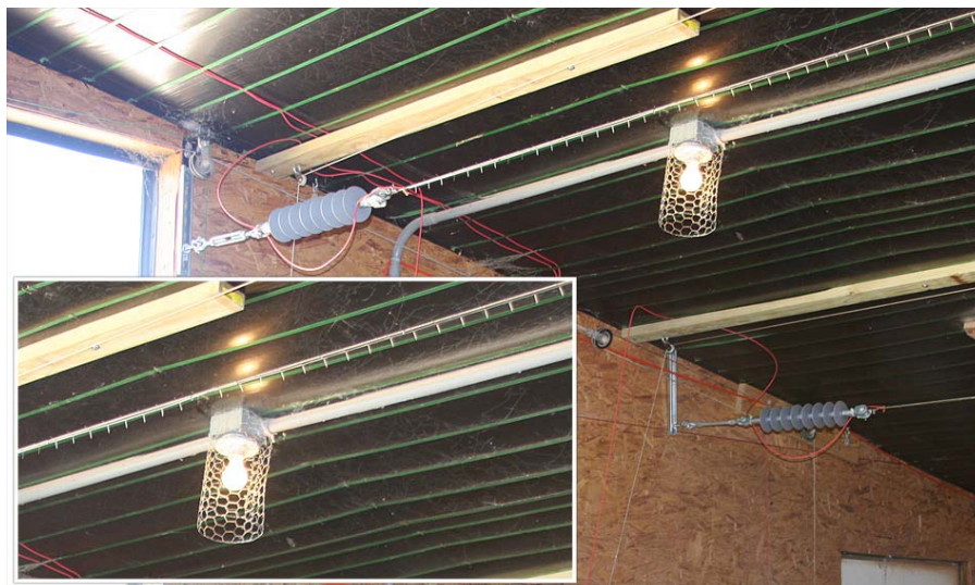
Figure 1. Corona lines running from power source.
